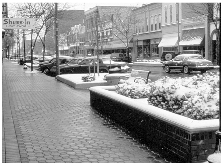
Figure 1. A snow melting system under concrete pavers in downtown Holland, Michigan has performed well since 1988.
