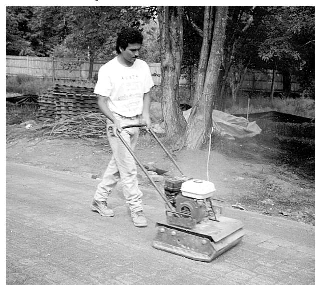
Figure 9. Final compaction of the pavers and settling of the sand into the joints.
